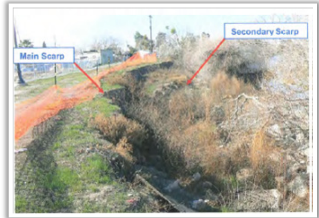
Landslide Adjacent to Firebaugh along San Joaquin River
