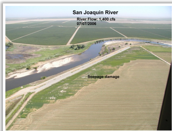
Seepage Damage along the San Joaquin River, 2006
