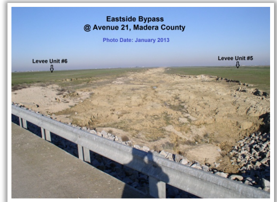
Eastside Bypass Scour Caused by Subsidence, 2013
