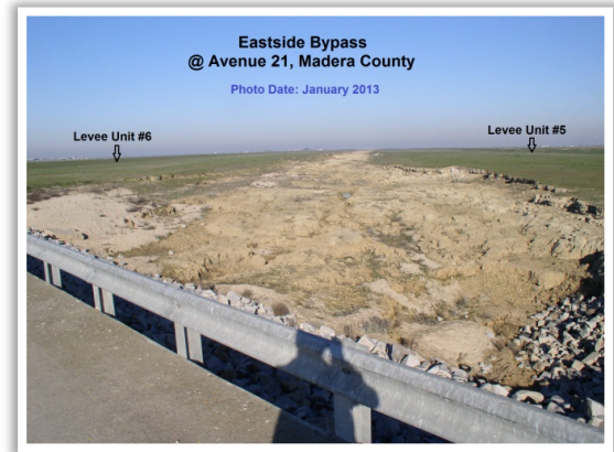
Eastside Bypass Scour Caused by Subsidence, 2013
